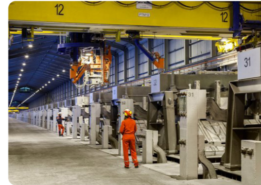
A serious incident occurred at Norðurál in the autumn, when transformer failures caused around two-thirds of the plant to shut down temporarily.
