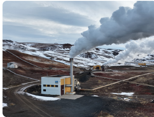
Major upgrades have been carried out at Bjarnarflag, Landsvirkjun’s oldest geothermal power station.
